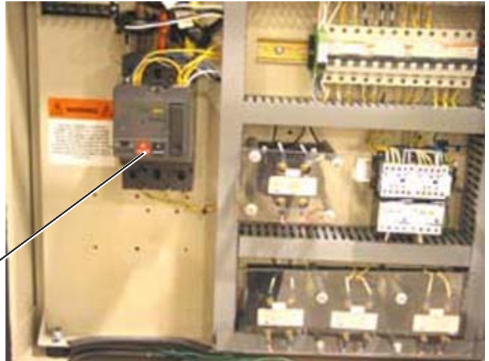
Generator Breaker (CB1)
