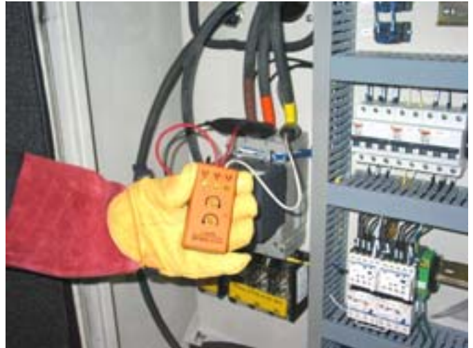
Rotation Meter Connected To Generator Power
