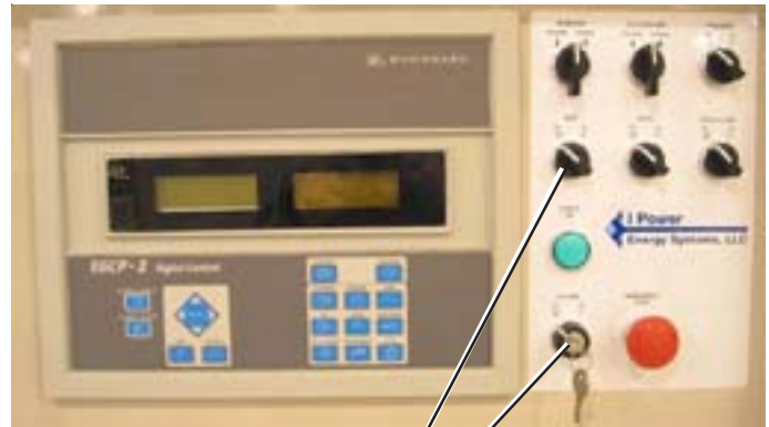
Test Switch System Switch
